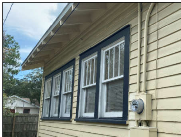
Figure 3: Example of typical reveal found in historic double-hung sash windows, 2734 2 nd Ave. N.
